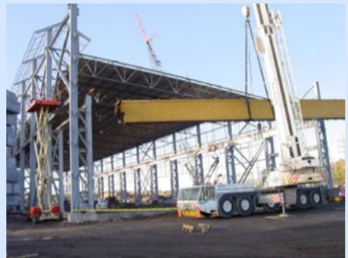
HAN-TEK helped its customer design a structure to house the larger-capacity billet cranes.
